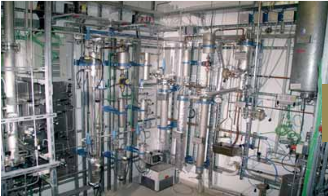
Hydroprocessing- Anlage der CUTEC Hydroprocessing plant at CUTEC
